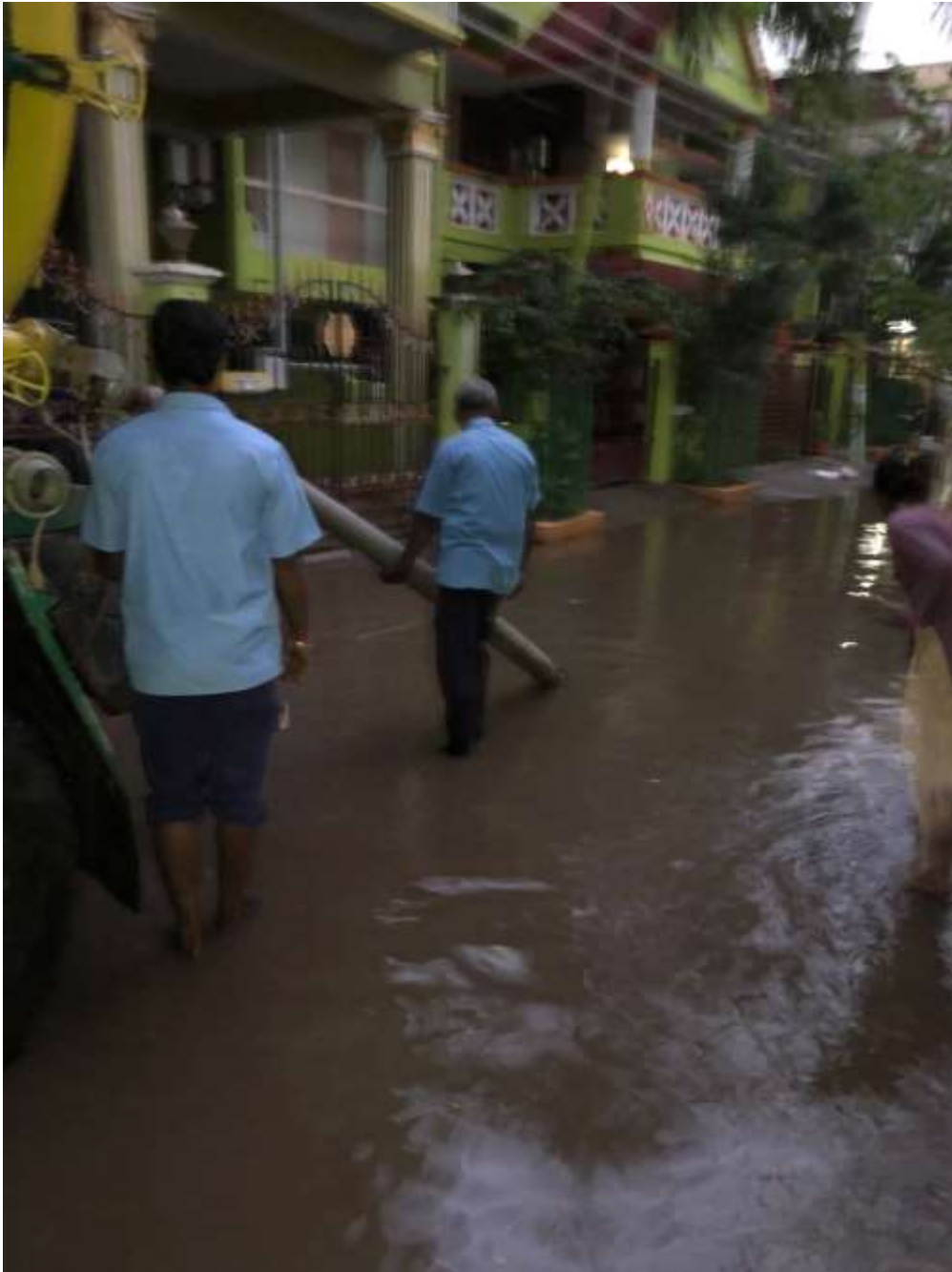
Dewatering stagnated rainwater using super sucker at MGR nagar 7th st avenue in Area XIII
