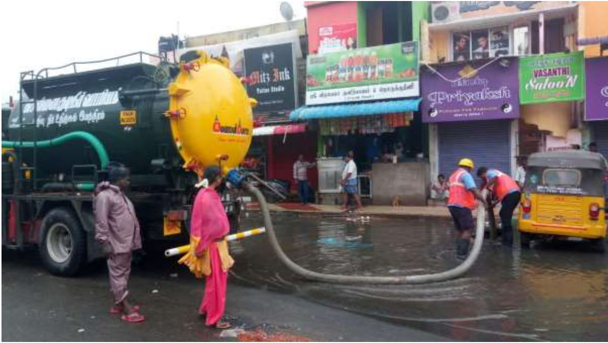
Dewatering stagnated rainwater using super sucker at 7th Avenue near Velankanni Church
