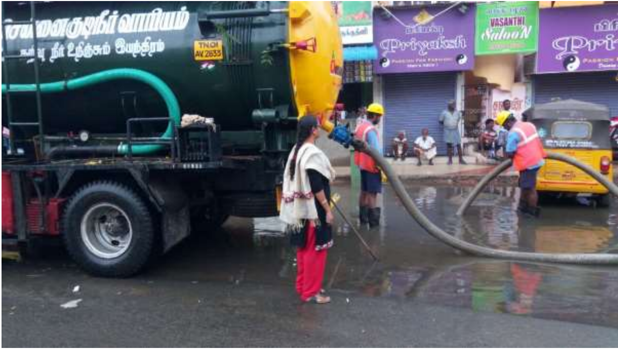
Area 13, Dewatering the stagnated water using Super Sucker at 7 th Avenue - Besant Nagar.
