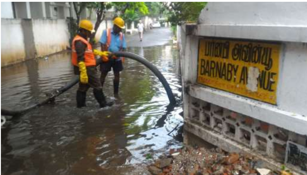
Area 8, Clearing stagnated rain water by using Super Sucker at Barnaby Road, Kilpauk.
